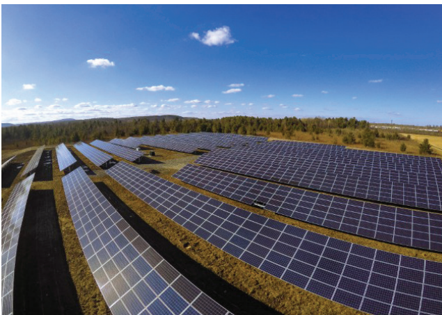
A 3.75-megawatt system installed at a former clay mine provides clean power for the Town of Bethlehem, New York.
