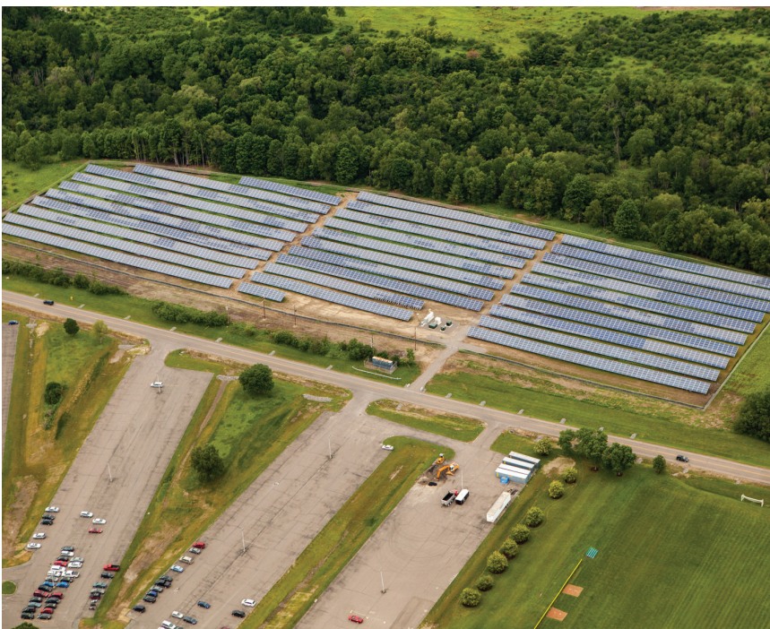
A 2.6-megawatt system at Tompkins Cortland Community College in Dryden, New York, provides 90 percent of the campus' electricity needs.
